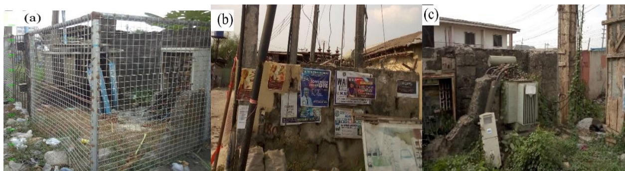
Figure 2. Locations Photos of Transformers (a) Enerhen (b) Ogbomoro and (c) Ekpan in Uvwie Local Government Area, Warri Metropolis
